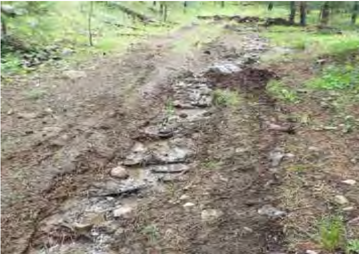
Figure 1 Note the erosion down the existing road
